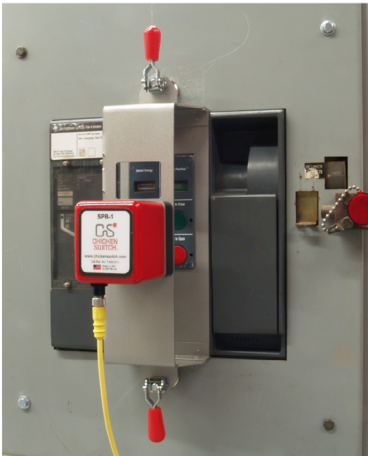
Picture A - SPB-1 shown installed on breaker
