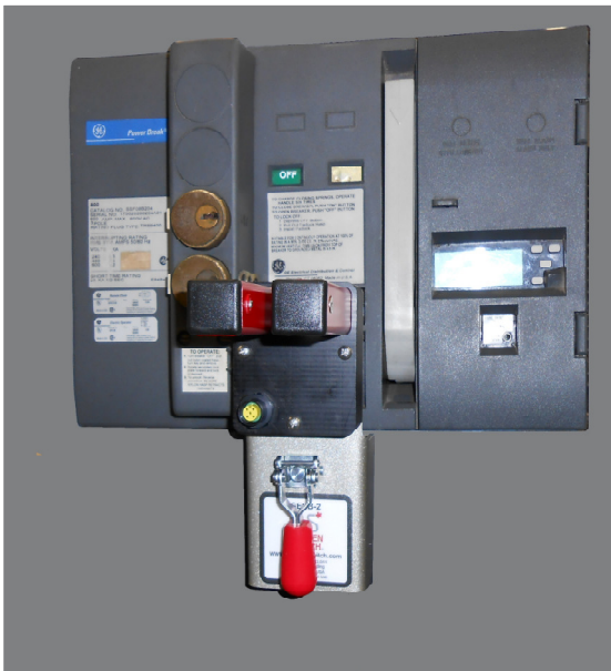
Picture A - GEPB-2 shown installed on breaker
